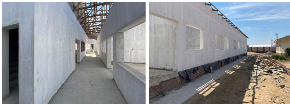
Fig. 2. New neonatal unit in Swakopmund: construction work is on hold until a new contractor can be found.
