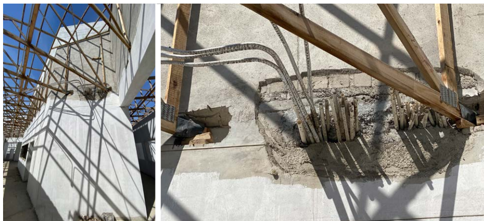
Fig. 3. New neonatal unit in Swakopmund: the roof is still not covered, and unprotected structures show signs of damage.
