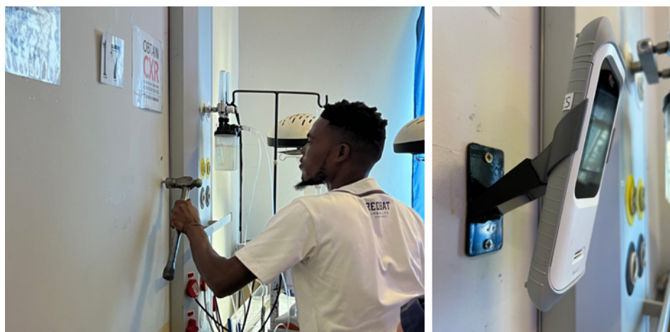
Fig. 14. The wall-mounted brackets for the Masimo® Rad-G pulse oximeters are installed in the Prem Unit at Rundu State Hospital.
