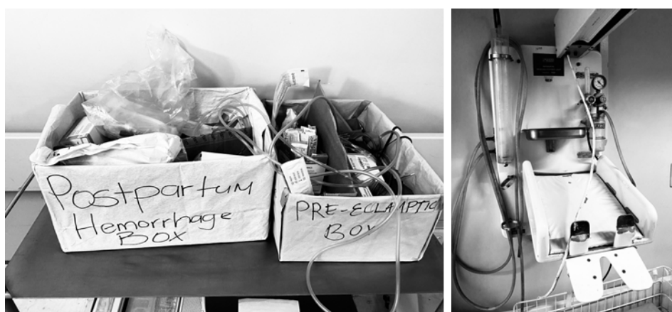
Fig. 7. Room for improvement: the labor and delivery ward at Katima Hospital continues to be poorly equipped (the wall-mounted neonatal resuscitation device on the right was no longer in use but had not yet been removed) and existing equipment is poorly maintained.
