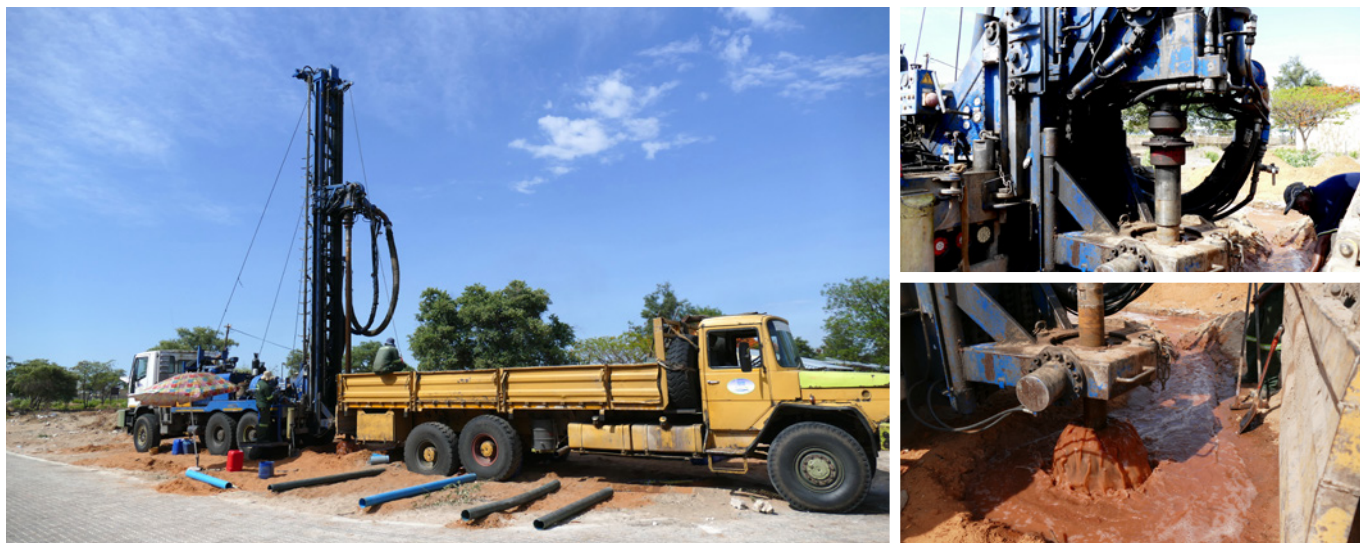
Fig. 11. Drilling for water on the hospital grounds in Rundu to secure uninterrupted water supply.
